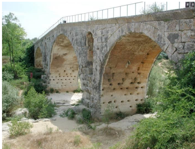
Figure 4 : The Julian bridge, on the Via Domitia. One can notice the holes made between the stone blocks, on the outside of the arches, to steal the iron staples used to bind the stones together.
