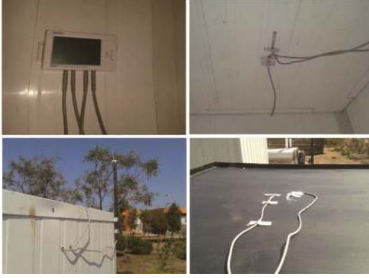
Fig. 4 Temperature sensors set-up
